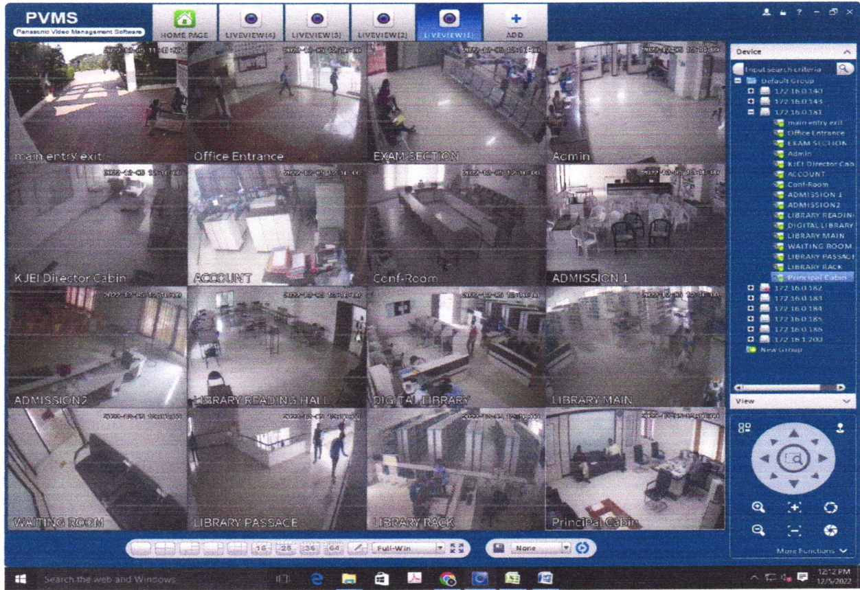
CCTV Cameras Used in College
